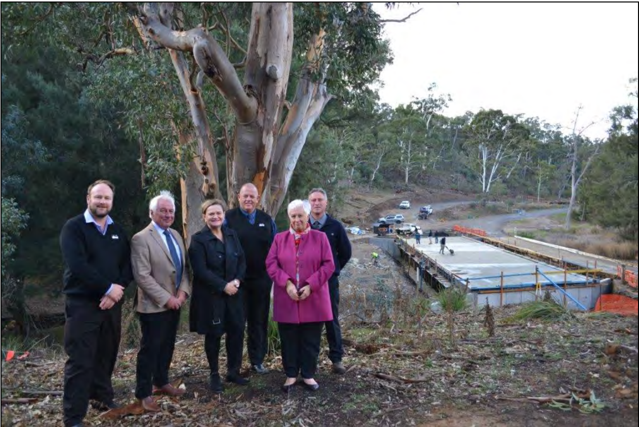
Member for Goulburn, Wendy Tuckerman MP with Oberon Shire Council Mayor and Upper Lachlan Shire Council Mayor and senior staff at the Oberon Road, Abercrombie River Bridge worksite
