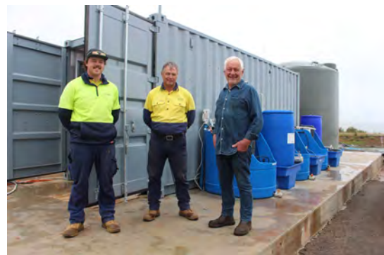
Mayor John Stafford with Council team members Lachlan Scott and Rodney Smith after the installation of the new Water Treatment plant at Taralga
