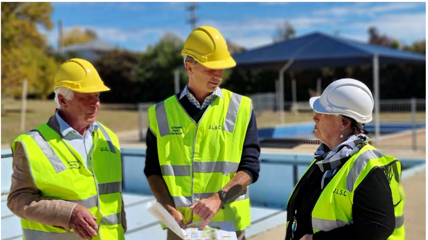
Mayor John Stafford with MP Angus Taylor and General Manager Colleen Worthy inspecting the MAAC project
