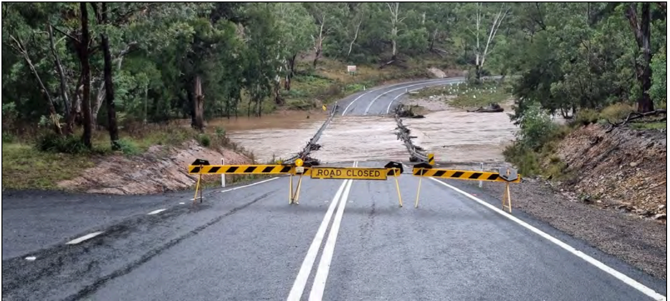
Flooding was prevalent in 2020/2021 – Abercrombie River Bridge on Oberon to Taralga Road MR256
